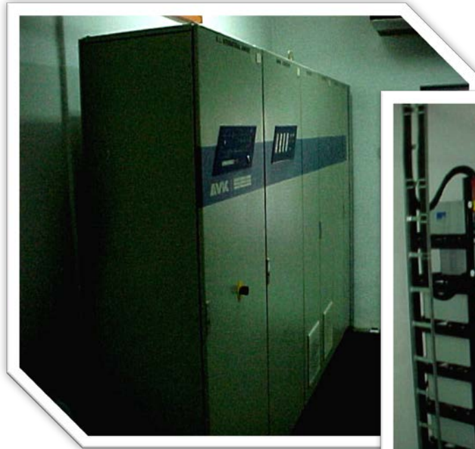
UPS Control Panel
