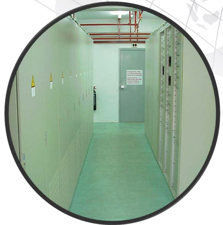
Transformer Module & Constant Current Regulator Panels
