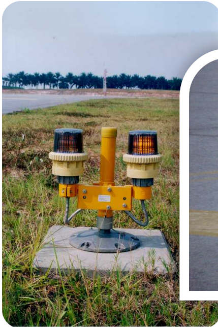
Traffic / Stop-Bar Guard Lights
