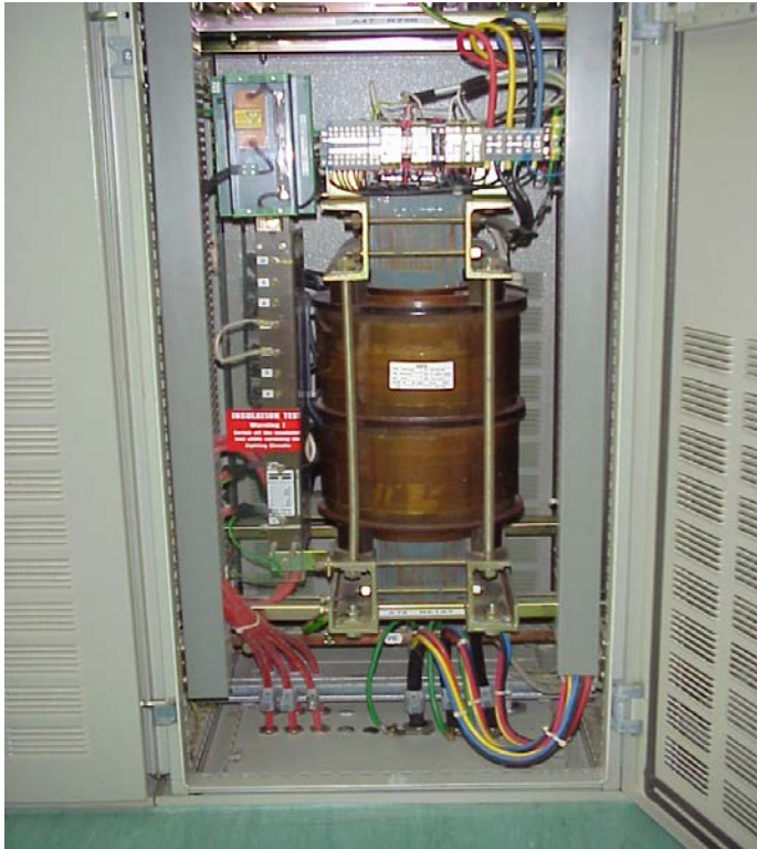
Transformer Module – 25KV
